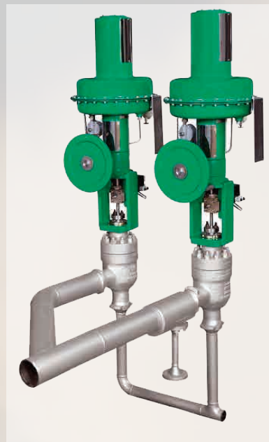
Fig. 8 DVL desuperheater installed at the outlet of main steam valve in a steam PRDS
